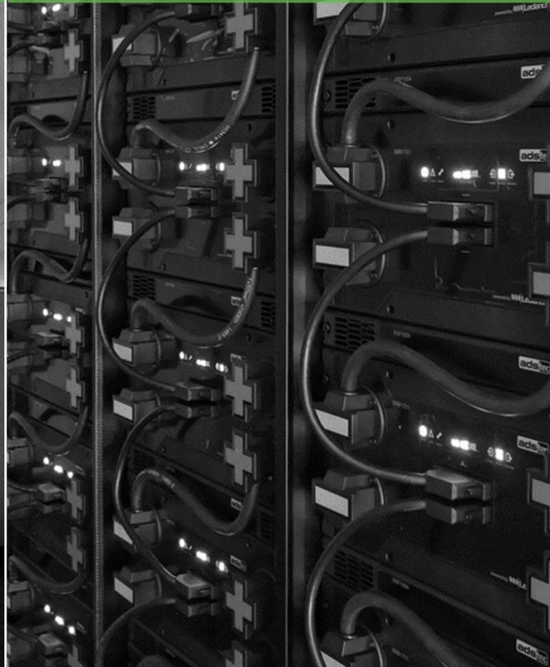
C&I Energy Storage Systems
